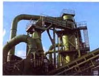
The shredder's dust extraction system ensures emissions are kept to within 15 milligrams per cubic metre.
